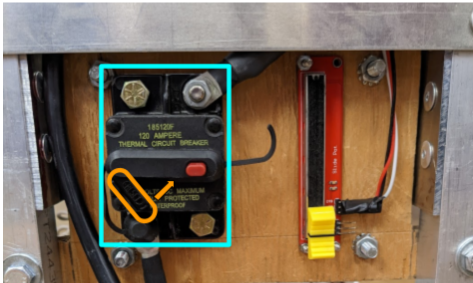
The back (controls) plate with the main breaker outlined in blue and the breaker arm outlined in orange with an arrow indicating how to power on.
